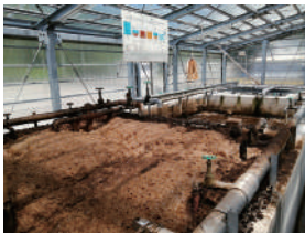
Wastewater treatment tank (aeration)
